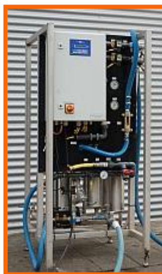
Nanofiltration / Reversed Osmose unit
