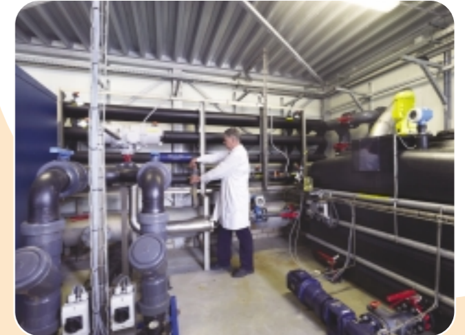
Post treatment MBBR FrieslandCampina Maasdam
